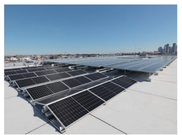
Photovoltaic power generation system constructed on the roof of a training facility "Sumitomo Densetsu Kawasaki Technical Center," which was opened in March 2023
